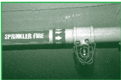
Install fire detection systems such as this sprinkler system with a sensor.
